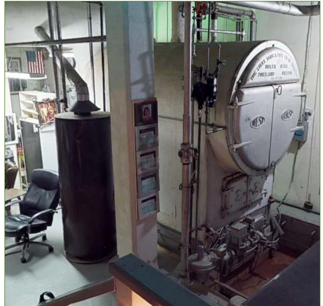
Lincoln HS Boiler
