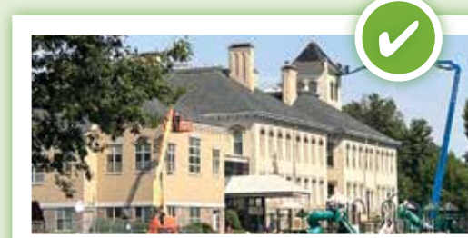
SK Mountain Construction put a new roof on historic Sharpstein Elementary this summer.
